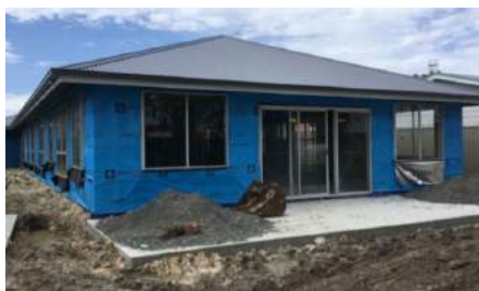
New beginnings on the Central Coast as the first foundations were laid for a new shared living home
